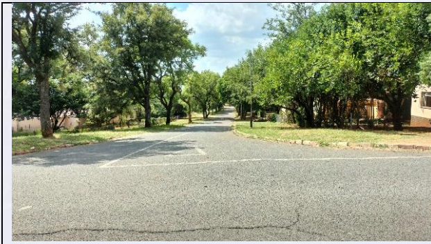
Figure 88: Transverse cracks on roads surface
