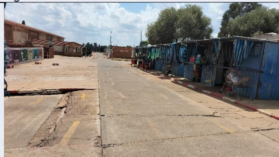
Figure 86: Concrete Pavement condition
