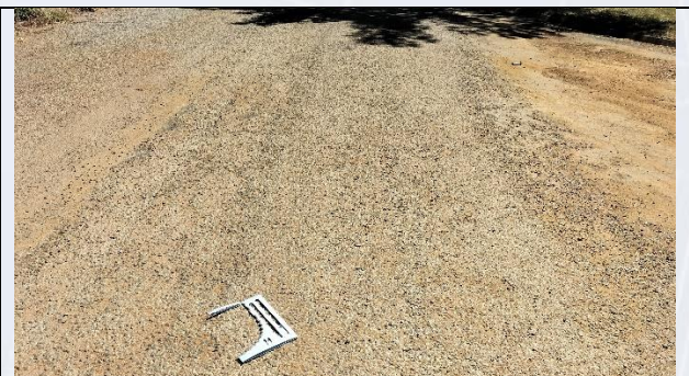
Figure 38: Evidence of poor stormwater management-siltation, in some cases
