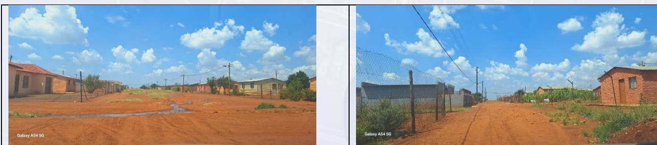
Figure 22: Conditions of gravel roads
