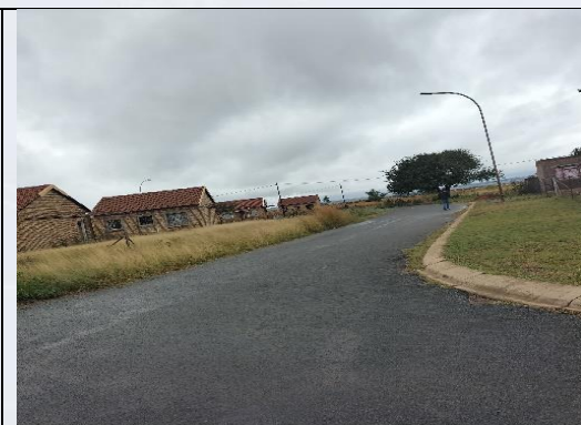
Figure 59: Condition of some roads; cross fall
