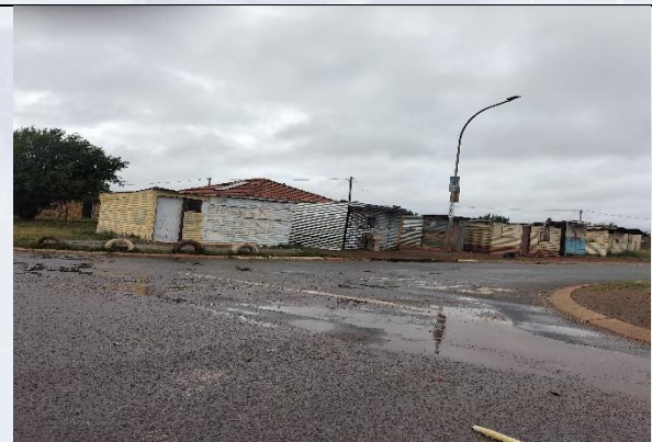
Figure 62: Stormwater deficits noted at most intersections noted
