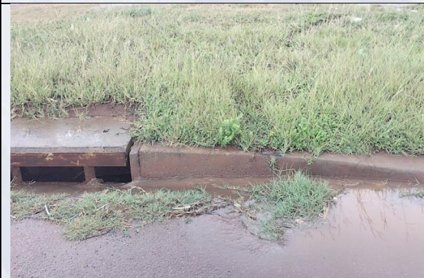
Figure 61: Kerb inlet working perfectly. Cleaning and clearing of the opening required
