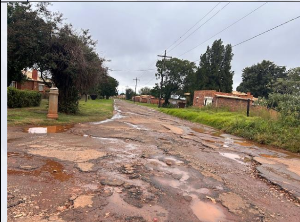
Figure 106: General surface condition of the roads
