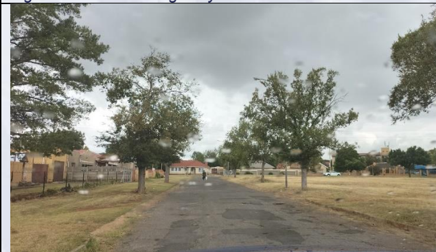
Figure 53: Road condition- cracking and pothole sealing
