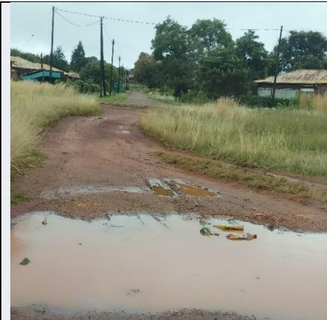
Figure 104: illegal roads being formed in a bid to avoid the poor roads
