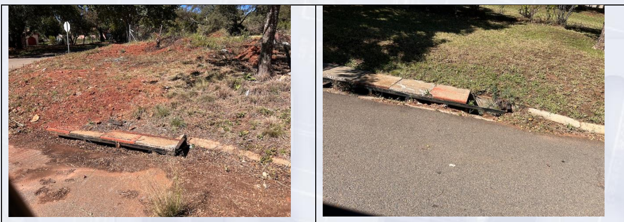
Figure 117: Clogged Kerb inlets
