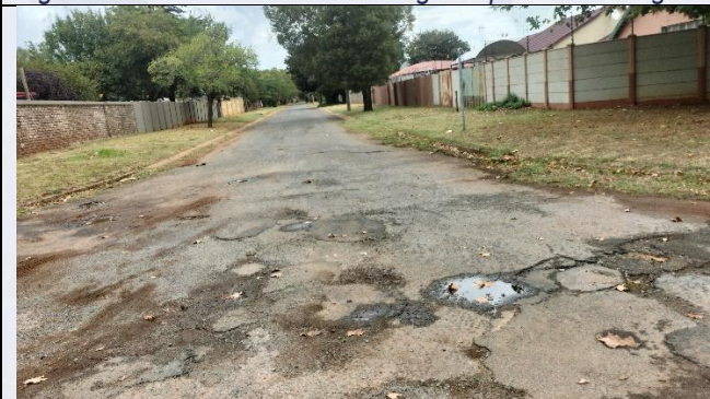
Figure 54: Road conditions on some of the worst street
