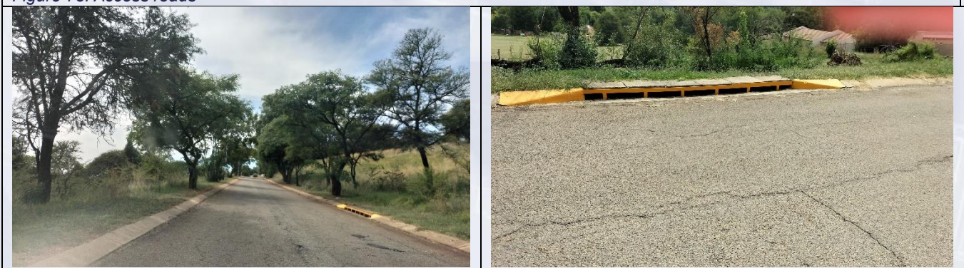
Figure 79: Stormwater structures-Kerb Inlet
