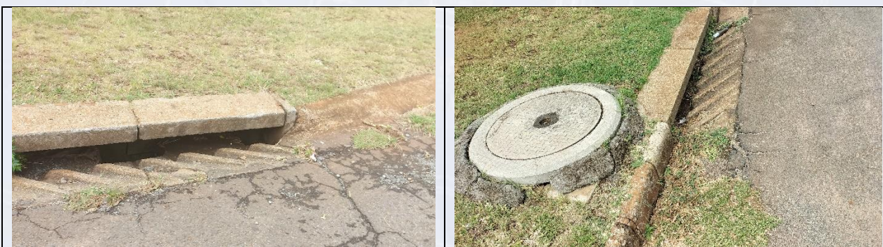
Figure 50:kerb inlets needing cover replacement and cleaning
