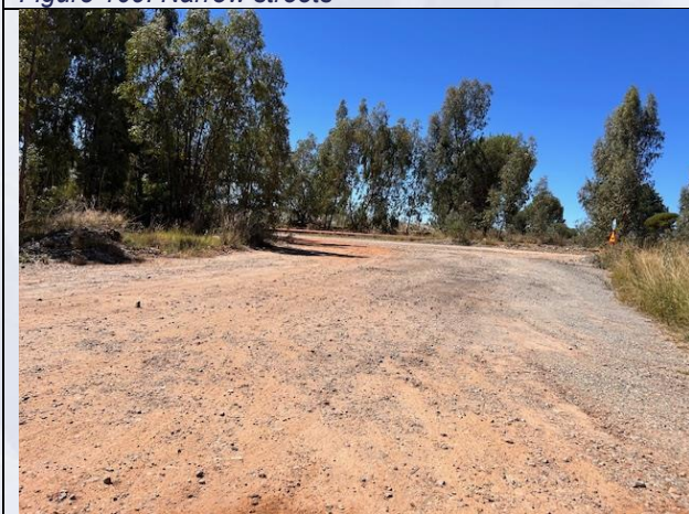
Figure 111: Road surface disintegration
