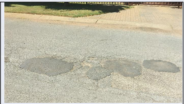
Figure 33: Evidence of scattered maintenance works
