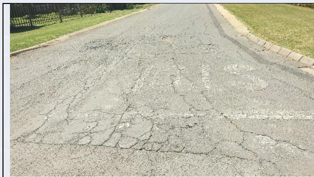
Figure 32: General condition of some street
