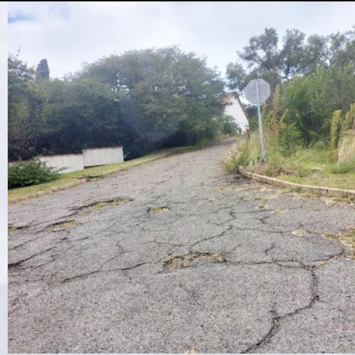
Figure 95: Some road condition on isolated portions
