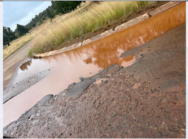
Figure 105: Stormwater was not catered for on all roads
